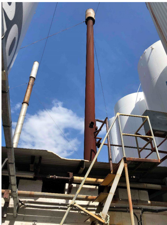
Image 1 – EPA 1 Thermal Oxidiser
